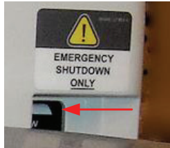
Figure 6-1: Breaker Position OFF
